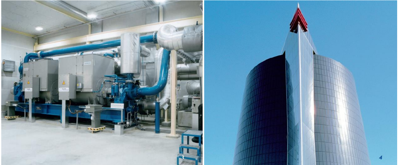
Fig. 40. Inside view of Lund's energy centre, and the buffer tank built for flexibility of district heating. Photos: Friothers AG and Lunds Energi AB.
