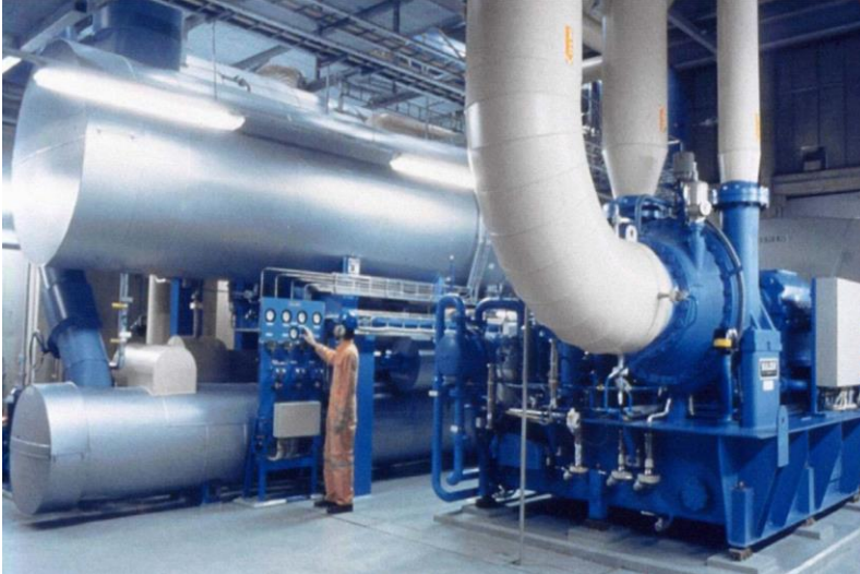
Fig. 41. Ropsten is the largest sea water heat pump facility worldwide, Värtaverket cogeneration power plant in Stockholm. Photo: Friotherm AG.
