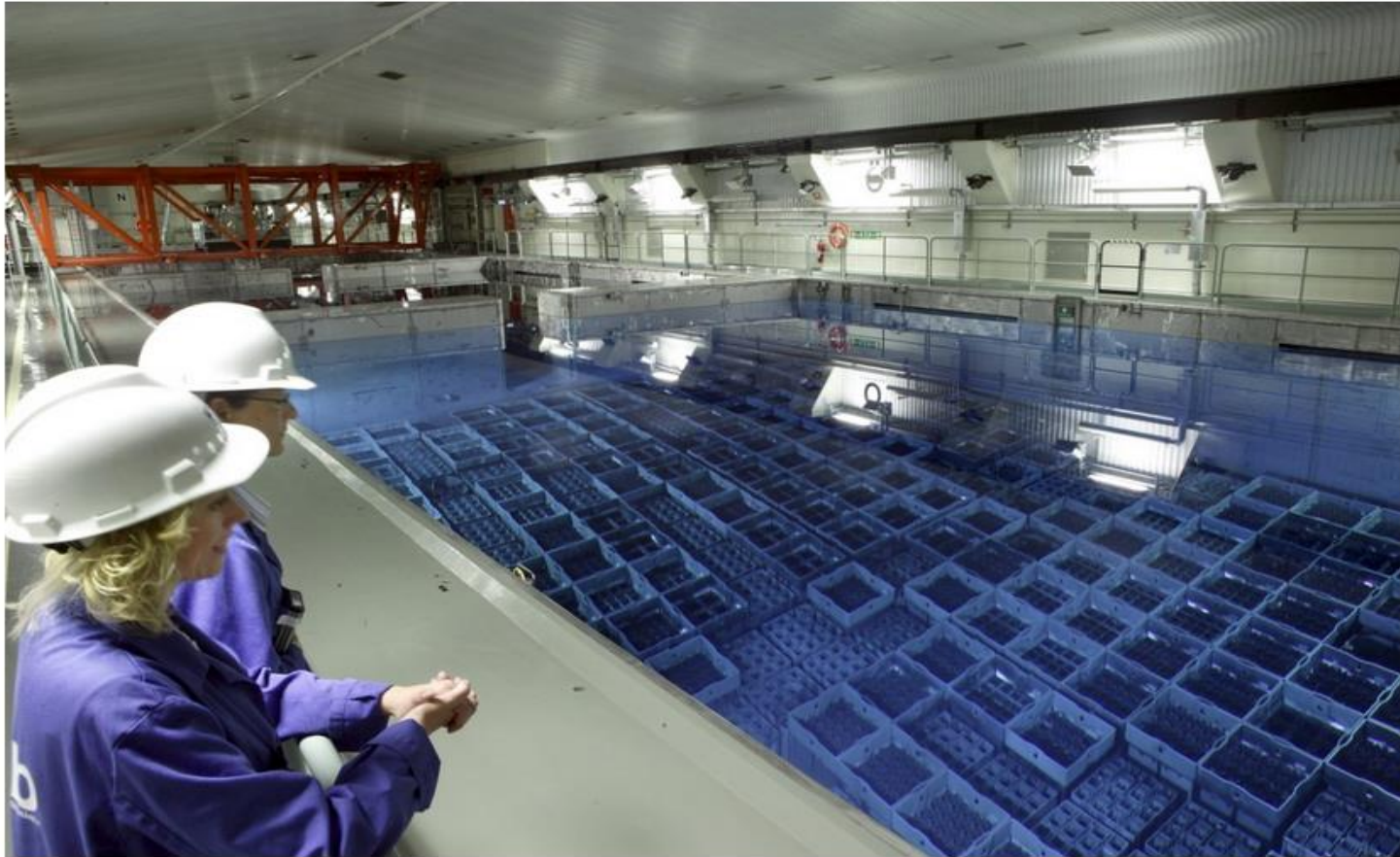
Central Interim Storage Facility (CLAB), Sweden. Image: SKB
